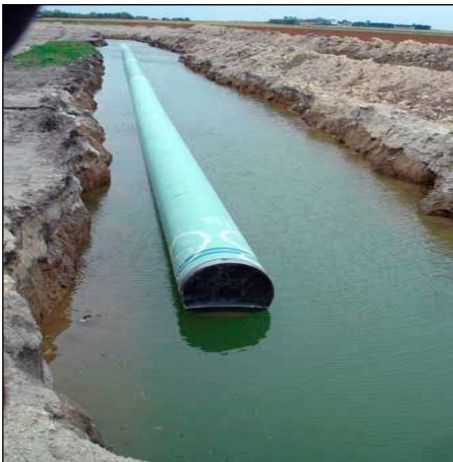
Landowners want tests to determine whether defective steel was used in the Keystone I tar sands pipeline running through the eastern Dakotas.
