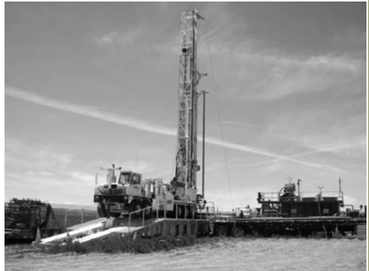
Drilling rig on platform with shakers for mud recirculation. Photo from Investigation of Ground Contamination near Pavillion, Wyoming DRAFT EPA 600/R-00/000 December 2011.
