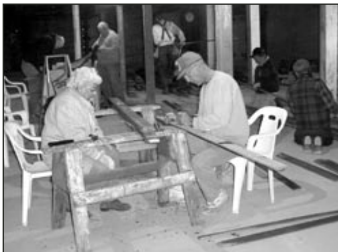
Volunteers are helping WORC and Northern Plains cut the cost of the office building by tens of thousands of dollars.
